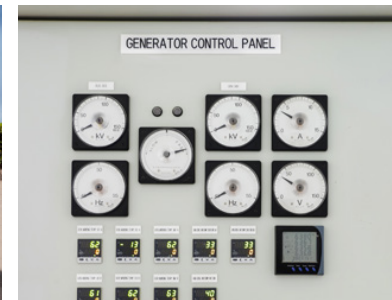
Dedicated space for Backup Generator Sets
